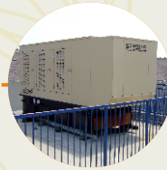
Power Backup for common area
